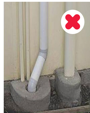
ORG connected to stormwater system
