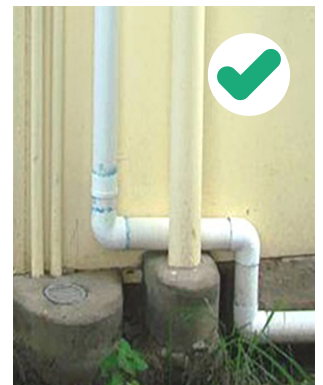
ORG connected to sewer network
